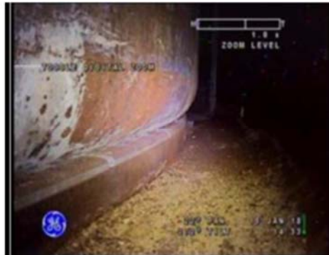
Tank AY-101 Annulus Floor Showing Debris
