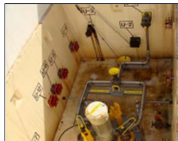
Typical Central Pump Pit
